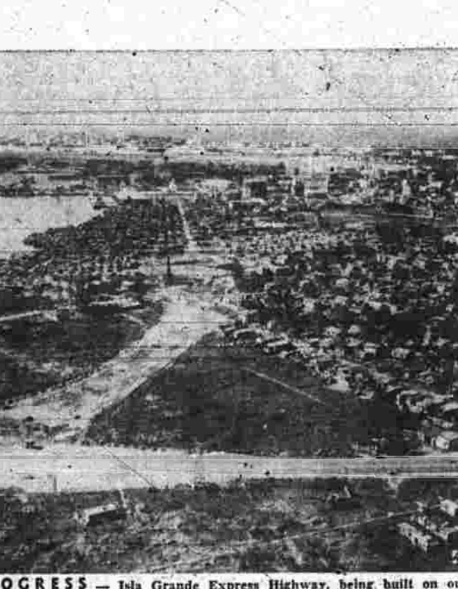
ROAD MARKS PROGRESS —Jala Grande Express Highway, being built on outskirts of San Juan, P. R., cuts through heart of slum area which will be cleared away by end of 1952.
